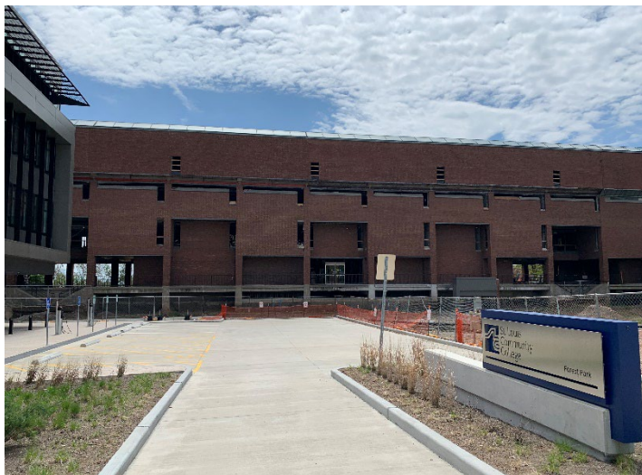
View of Towers A and B, the easternmost building sections of the St. Louis Community College – Forest Park, with interior demolition underway and new entry drive perpendicular to the original building, April 27, 2020 photo by John C. Guenther, FAIA, LEED AP
