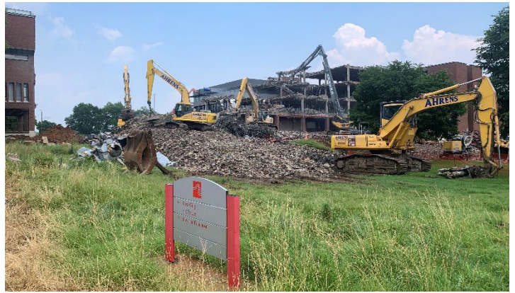
View of demolition of Towers A and B, July 7, 2020 photo by John C. Guenther, FAIA, LEED AP
