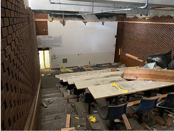
A periodical table of elements sign is one of the few educational items left amid debris in room A-110, a science lecture hall being prepared for demolition. (Photo by Markell Tompkins) The Scene, March 6, 2020 15
