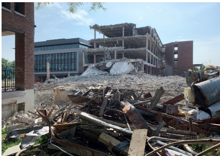
View of demolition of Towers A and B, July 3, 2020 photo by John C. Guenther, FAIA, LEED AP
