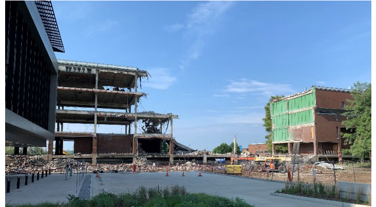
Towers A and B under demolition. July 3, 2020 photo by John C. Guenther, FAIA, LEED AP
