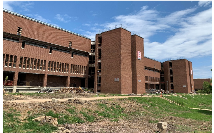
View of Towers A and B of the St. Louis Community College – Forest Park, with interior demolition materials on south lawn, April 27, 2020 photo by John C. Guenther, FAIA, LEED AP
