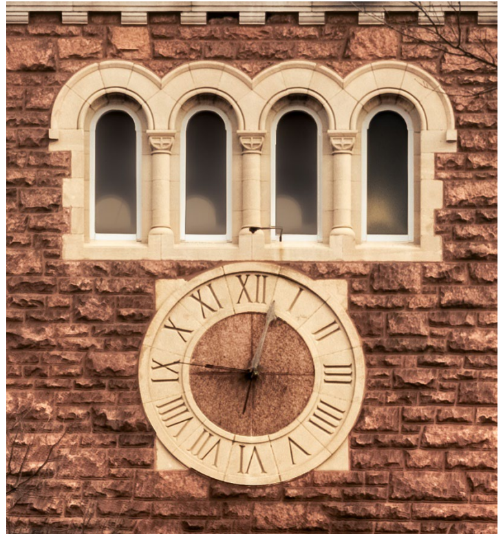
Pilgrim Congregational Church, clock face on tower is arranged as a circle over a recessed square. The design may have been referencing overlaid squares and circles as a symbol of harmony. Photograph © Andrew Raimist.
